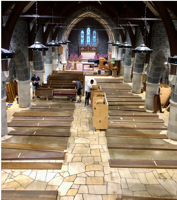
The pieces of the pews laid out on the floor prior to assembly.
