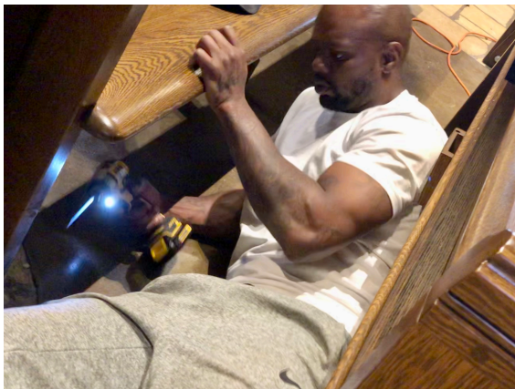
Every pew had to be screwed into the floor, a job for young, nimble and flexible workers.
